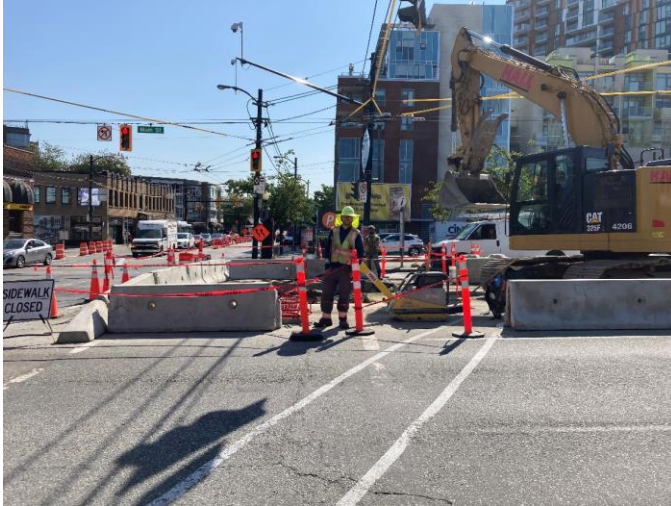
Main and 8th Utility Relocation Work: backfilling the excavation with the Main and Broadway intersection
