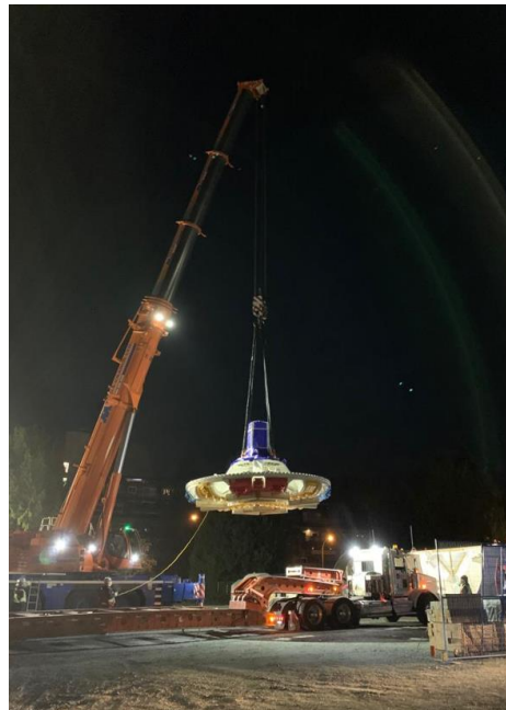
Arrival of the first cutterhead, which is the very front of the TBM.
