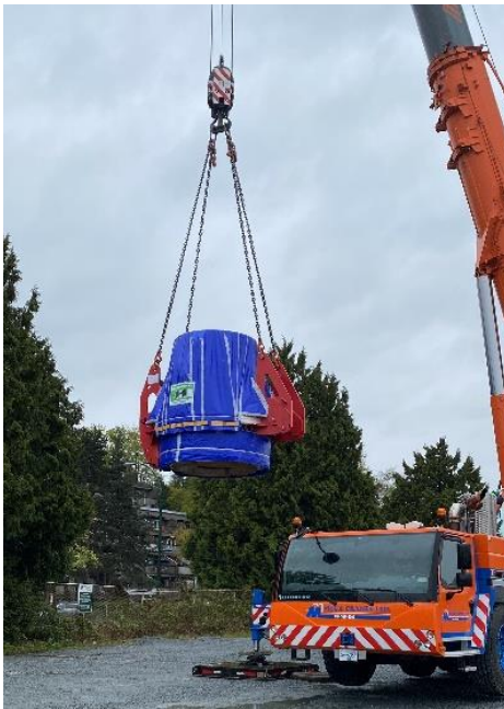
This main drive was the first component to be transported to the site! This is the mechanism inside the TBM that turns inside the cutterhead.
