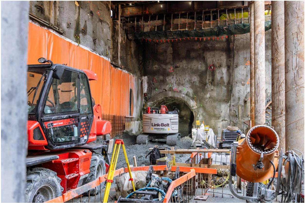
Figure 7: Arbutus Station: Progressing with excavation for the mined tunnels for the tail track.
