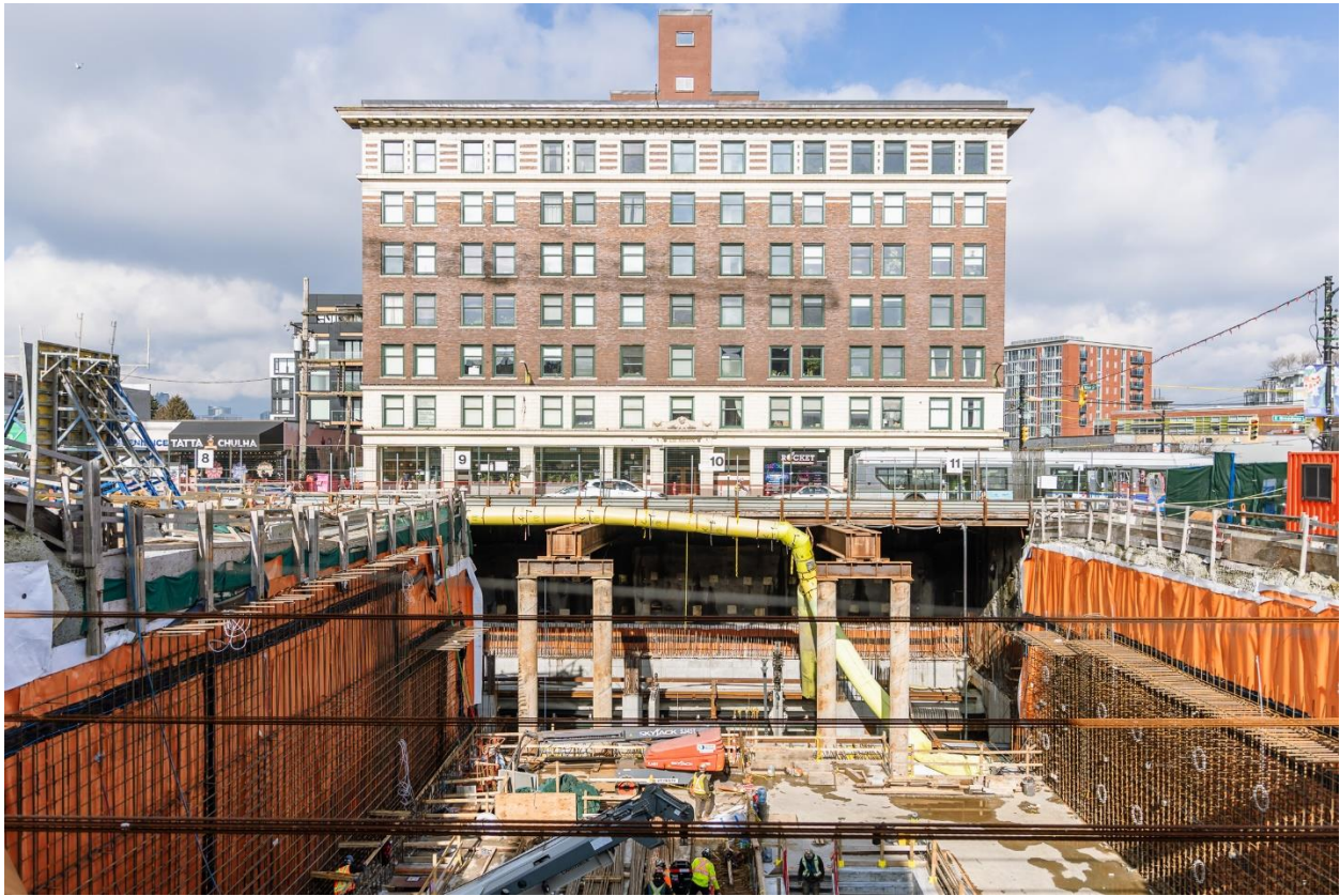
Figure 3: Mount Pleasant Station: Progressing with installation of rebar and concrete pours for the concourse-level walls in the headhouse.
