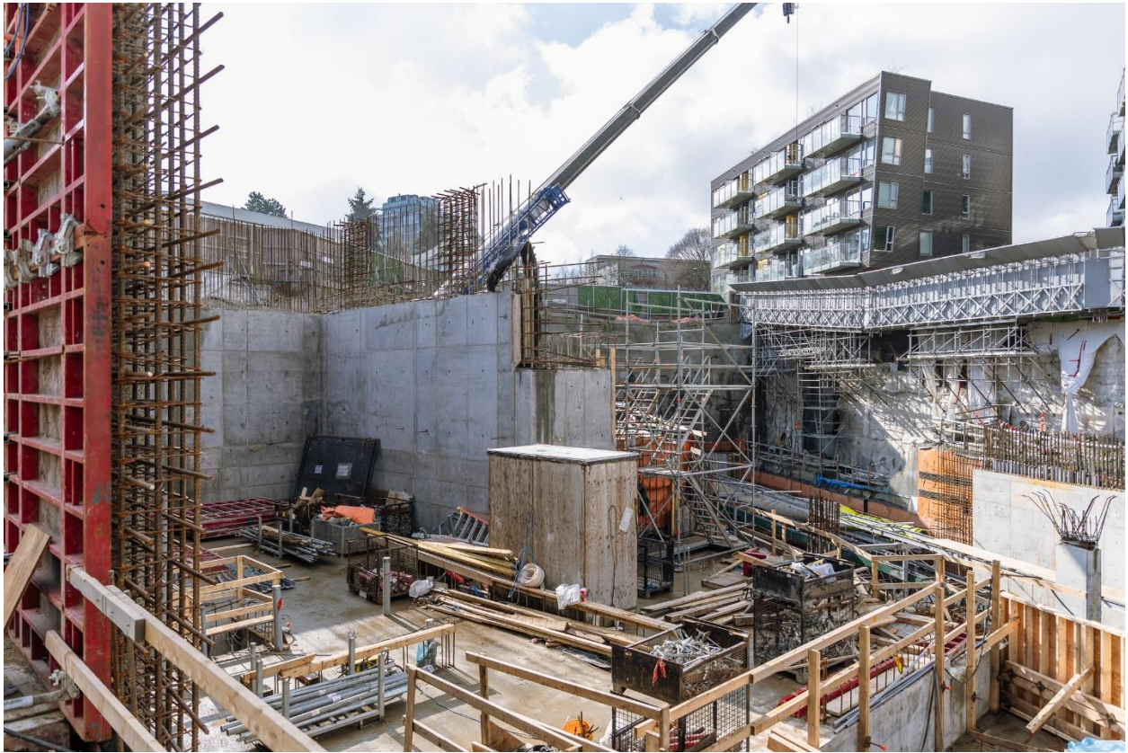
Figure 2: Great Northern Way-Emily Carr Station: Progressing with construction of the headhouse walls.
