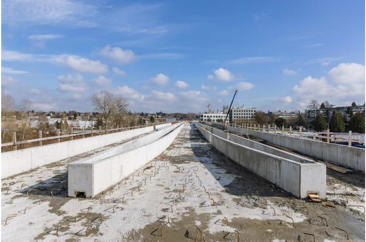
Figure 1: Elevated Guideway: Progressing with the construction of the parapets on the elevated guideway deck.
