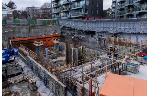
Figure 2: Great Northern Way-Emily Carr Station: Progressing with construction of the concourse-level columns and walls.
