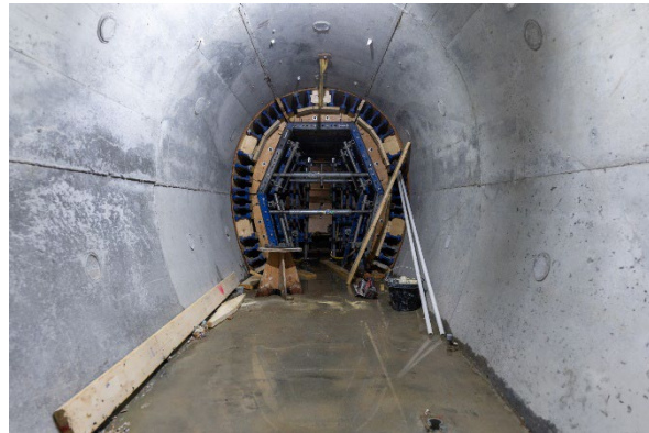
Figure 8: Tunnels: Progressing with construction of the cross passages that connect the two SkyTrain tunnels.
