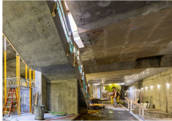
Figure 6: South Granville Station: Progressing with construction of the staircases connecting the platform and concourse levels.
