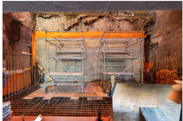
Figure 4: Broadway-City Hall Station: Progressing with construction of the passenger connection to the Canada Line northbound platform.
