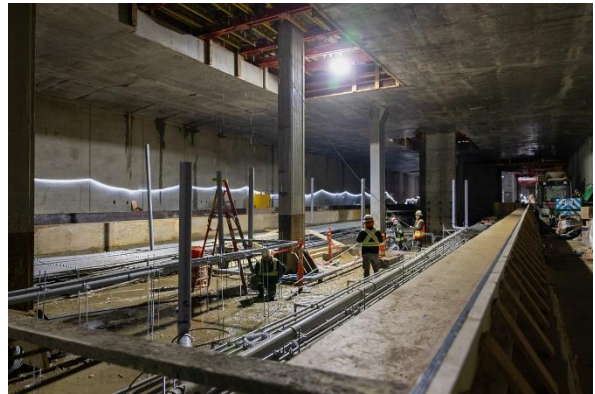
Figure 4: Broadway-City Hall Station: Progressing with rebar and conduit installation for the station platform.
