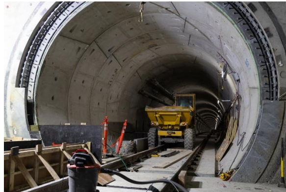
Figure 6: South Granville Station: Progressing with construction of the expansion joint cover plates.
