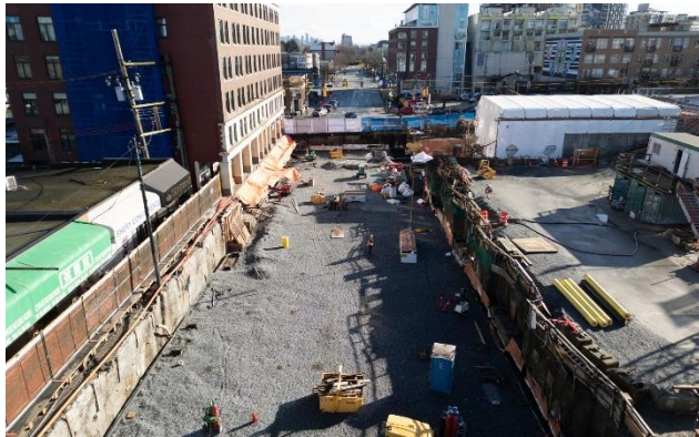
Figure 3: Mount Pleasant Station: Completion of traffic deck removal and progressing with backfill and utility work.
