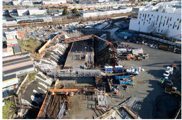
Figure 2: Great Northern Way-Emily Carr Station: Progressing with waterproofing the underground station roof.
