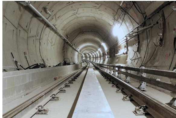
Figure 8: Tunnels: Progressing with Installation of the Linear Induction Motor (LIM) rail and power rail inside the westbound tunnel.
