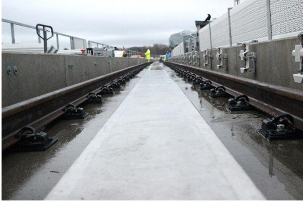
Figure 1: Elevated Guideway: Progressing with installing the power rail on the eastbound track
