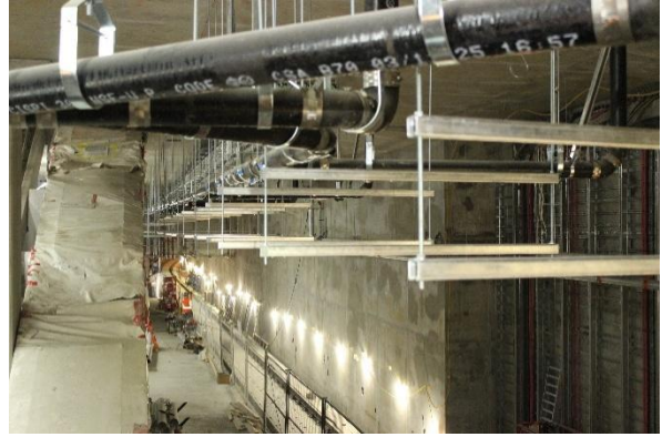
Figure 2: Great Northern Way-Emily Carr Station: Progressing with mechanical, electrical and plumbing installation inside the station.
