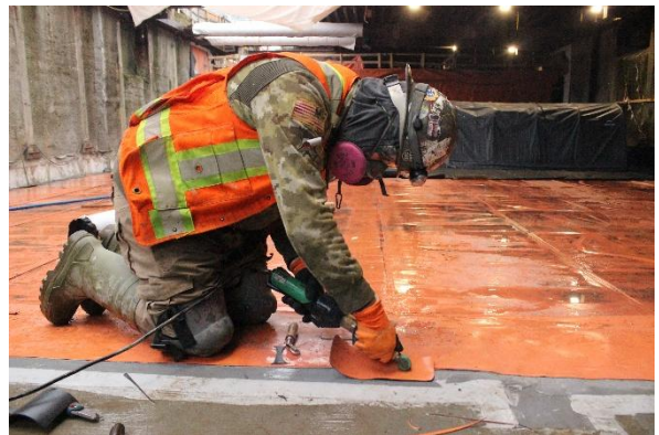
Figure 4: Broadway-City Hall Station: Progressing with waterproofing the station box and west shaft roof slabs.
